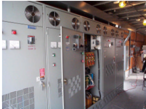
Figure 8: Five 100 HP motor control units shared between ten motors.
